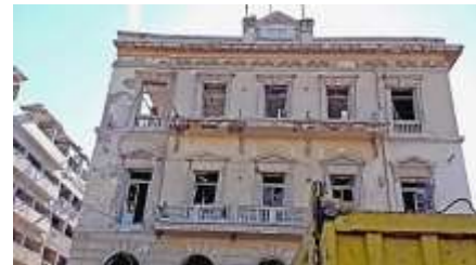
Pic (22): The fully destroyed front Façade in 2014
